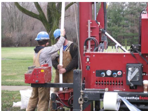
Monitoring well being installed as early warning system to protect Enon's drinking water
