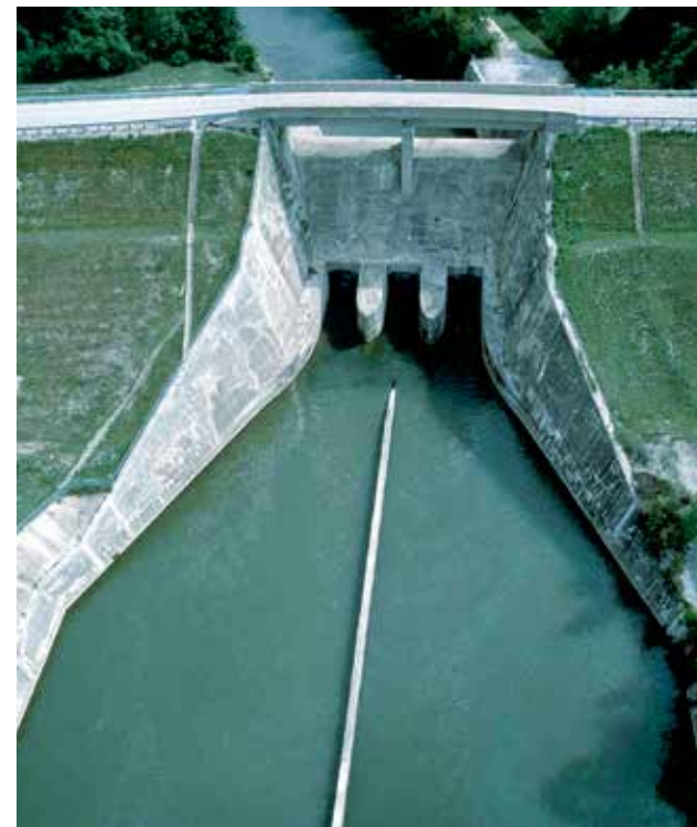
Huffman Dam near Wright Patterson Air Force Base is one of MCD's five flood protection dams.
