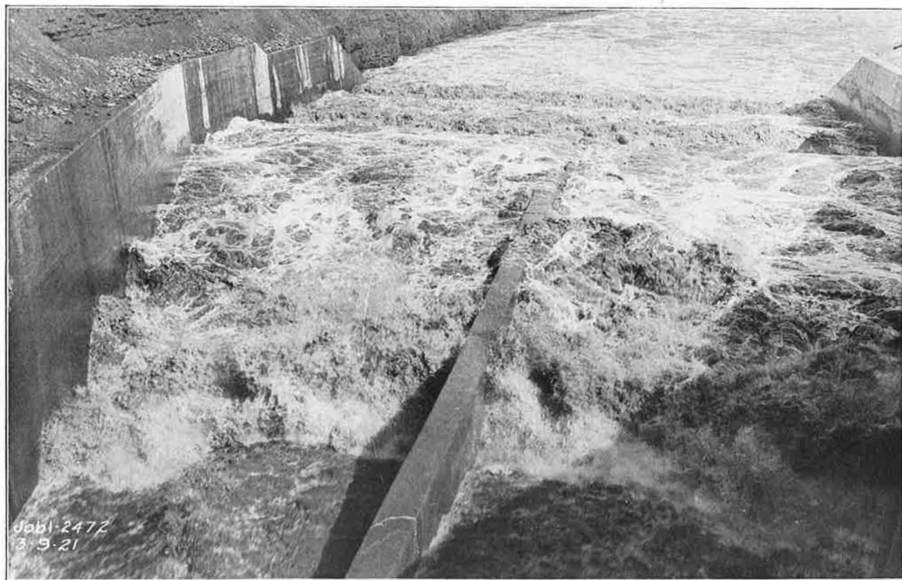
FIG. 290—GERMANTOWN CONDUIT OUTLET BASIN, FLOOD OF MARCH 9, 1921
