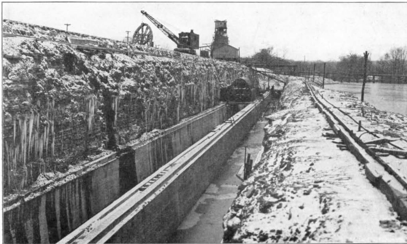
FIG. 79—THE CONDUITS AT ENGLEWOOD, DECEMBER 26, 1918.
