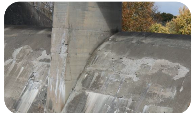
Deteriorating concrete of an emergency spillway
